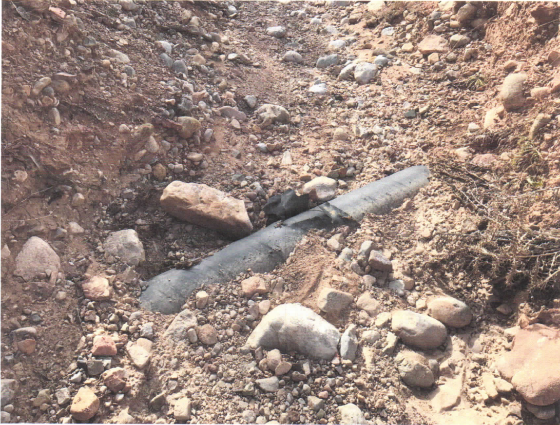
Exposed, damaged Enterprise High Pressure Natural Gas Liquids (NGL) Pipeline in a Small Creek Near Camino De La Rosa Castilla.
