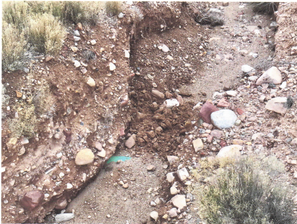
A Second Exposed Enterprise High Pressure NGL Pipeline in a Creek.
